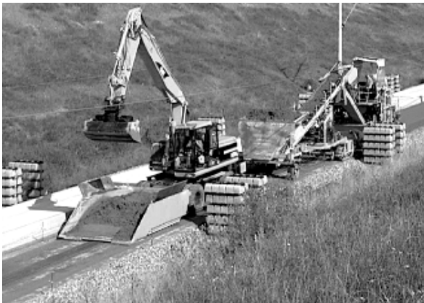
Fig. 9: Construction of a continuously reinforced concrete rigid track for a German high speed railroad with a slipform paver, delivering the concrete from the front of the paver
