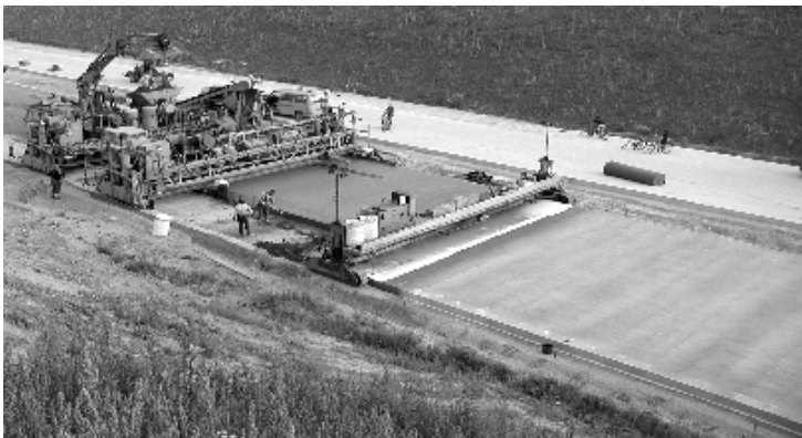
Fig. 10: Changing construction width during construction of a concrete pavement in slipform technique, behind the slipform paver the working platform follows for dragging a burlap to texture the wet concrete surface and to spray the liquid curing compound on the surface
