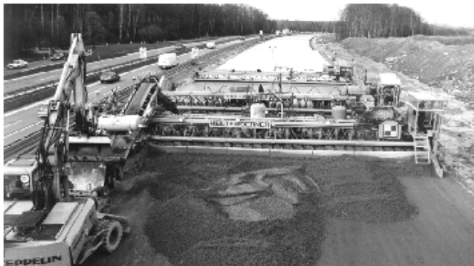
Fig. 8: Construction of a concrete pavement in two layers or two courses with two slipform pavers, the concrete for the top course / layer is placed in front of the second paver by a front-end feeder
