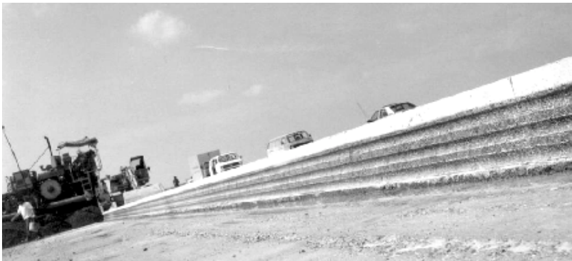
Fig. 12: Longitudinal construction joint of a "pilot strip" with sinusoidal profile, constructed with a slipform paving train, placement width 15 m
