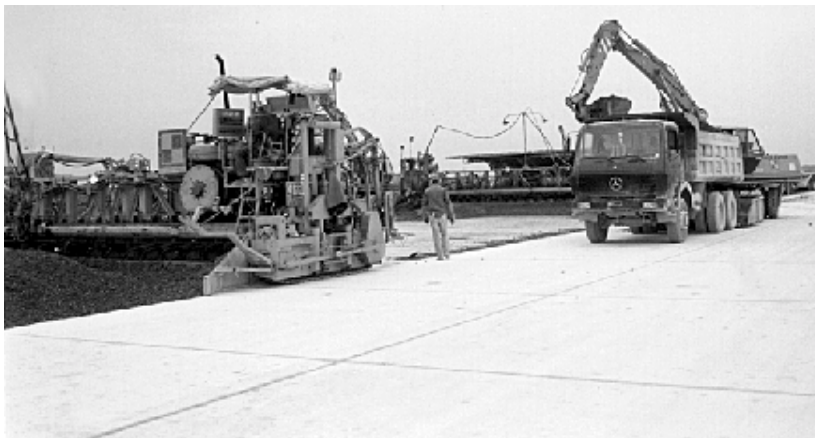
Fig. 8: Construction of the concrete pavement of the runway in two layers with a special slipform paving train consisting of two slipform pavers; here unloading the top concrete from trucks and spreading in front of the second paver by an excavator
